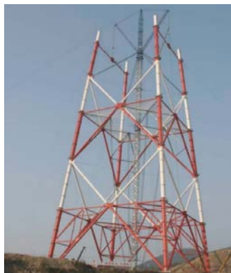
Figure 3. Electric transmission line tower in Zhejiang Province (Chen et al 2015)
